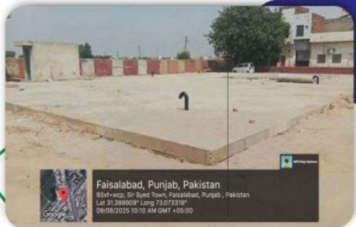
Fig 11: Stormwater Storage Tank at Dijkot Road, Faisalabad
