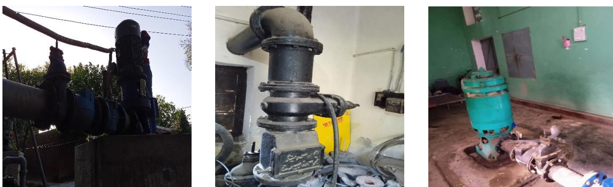
Figure 5: Sample pictures from field audit of pumpsets
