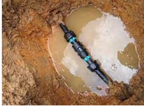
Figure 4-2 HDPE pipe joints leaking
