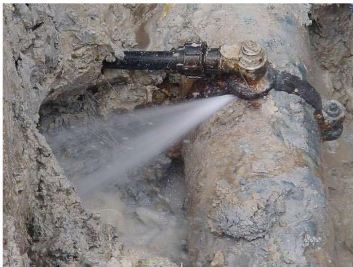
Figure 8-2 Small leaks go undetected
