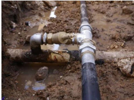
Figure 4-3 Pipe leaking underground
