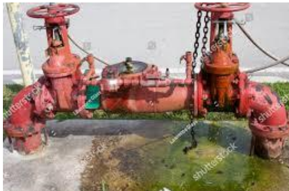
Figure 3-3 Packing Leaking of a Gate Valve
