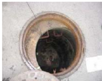
Offset of manhole block
