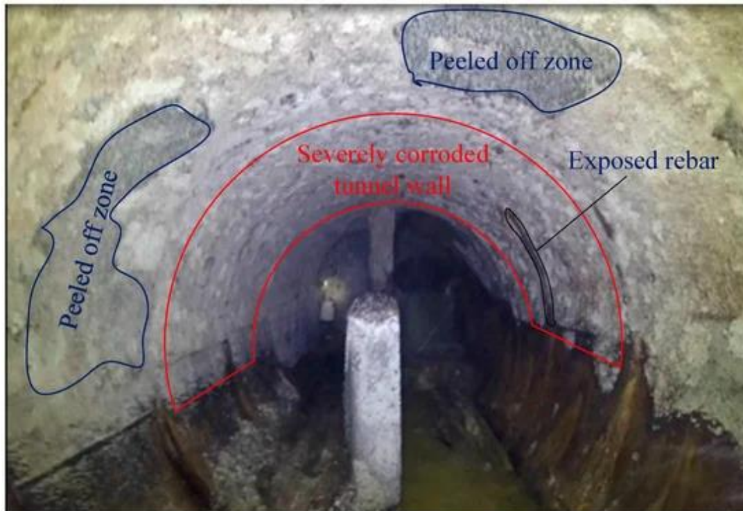
Figure 1-13 Sewer deterioration due to Corrosion
