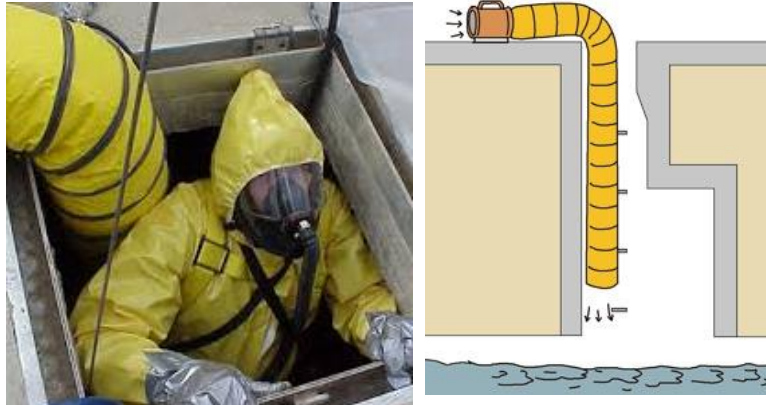
Figure 3-6 Fresh air should be supplied to the working location and the blower fan must be carefully located to avoid sucking in contaminated air.
