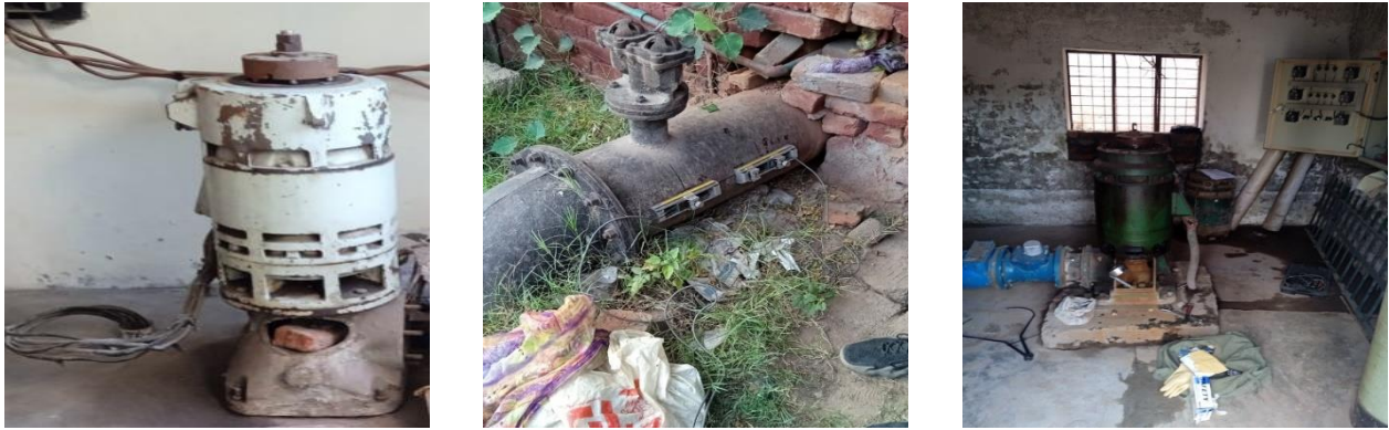
Figure 5: Sample pictures from field audit of pumpsets
