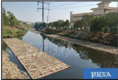
Lahore: (A) PMDFC has successfully installed floating wetlands in the Hudaira Drain. PUNA
